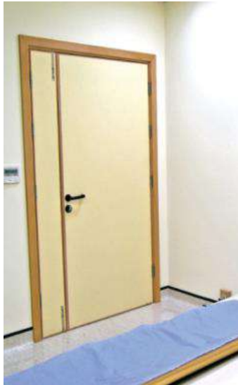
Lead Lined door
